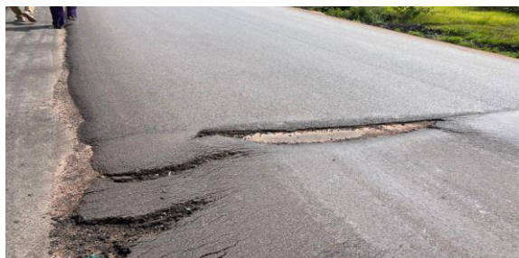
Fig1: Road eroded due to poor quality of delivery (AMG 2026)
